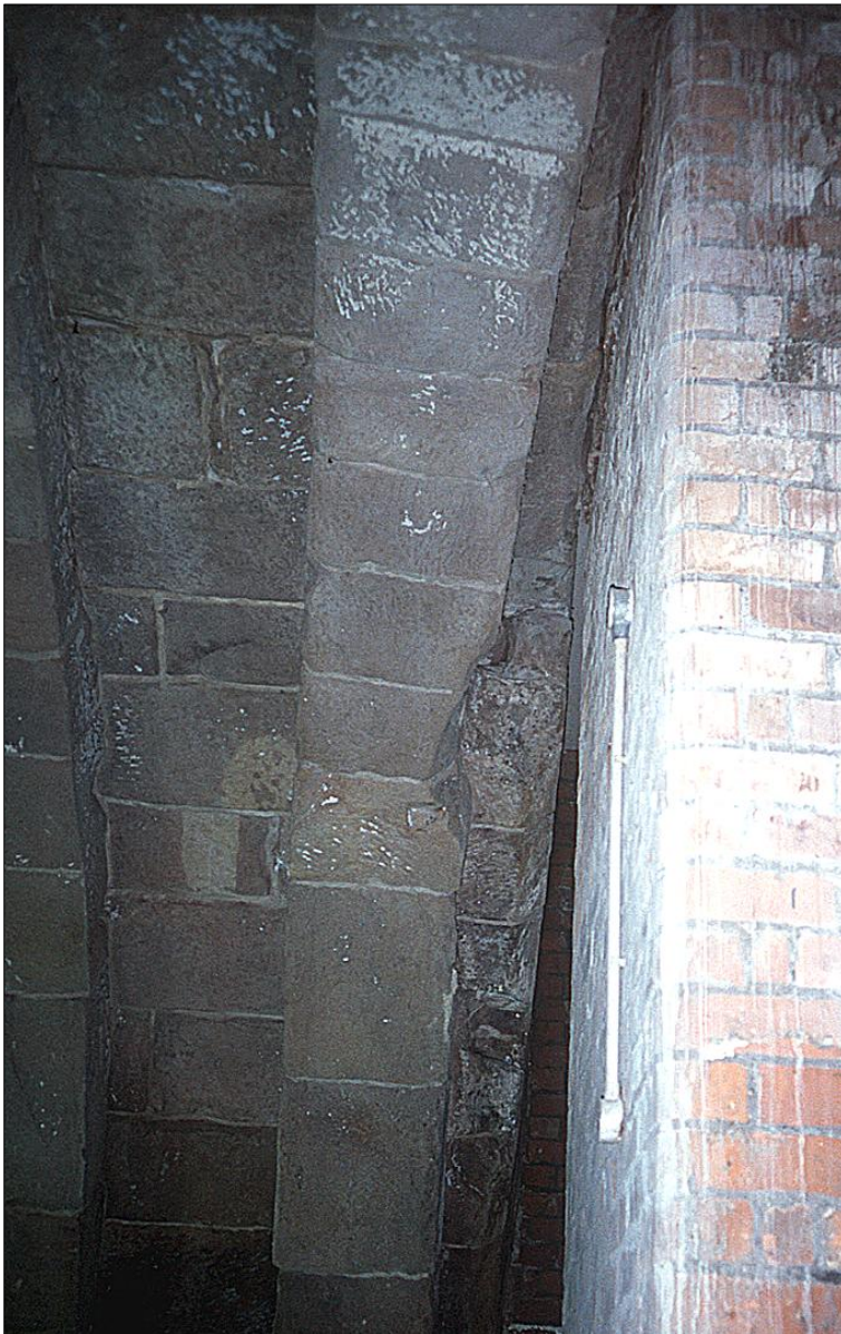
III B23: The south arch, the head of the western opening viewed from below, showing distortion of the stonework.
