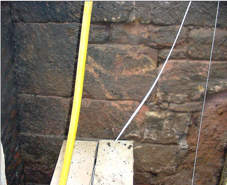
III B32: Stonework towards the north end of the east elevation butting onto soils (lower right).
