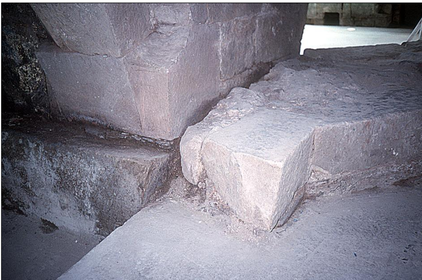
III B26: The north side of the south arch, detail of the base of the eastern rib (left), with the 'cutwater' on the right.
