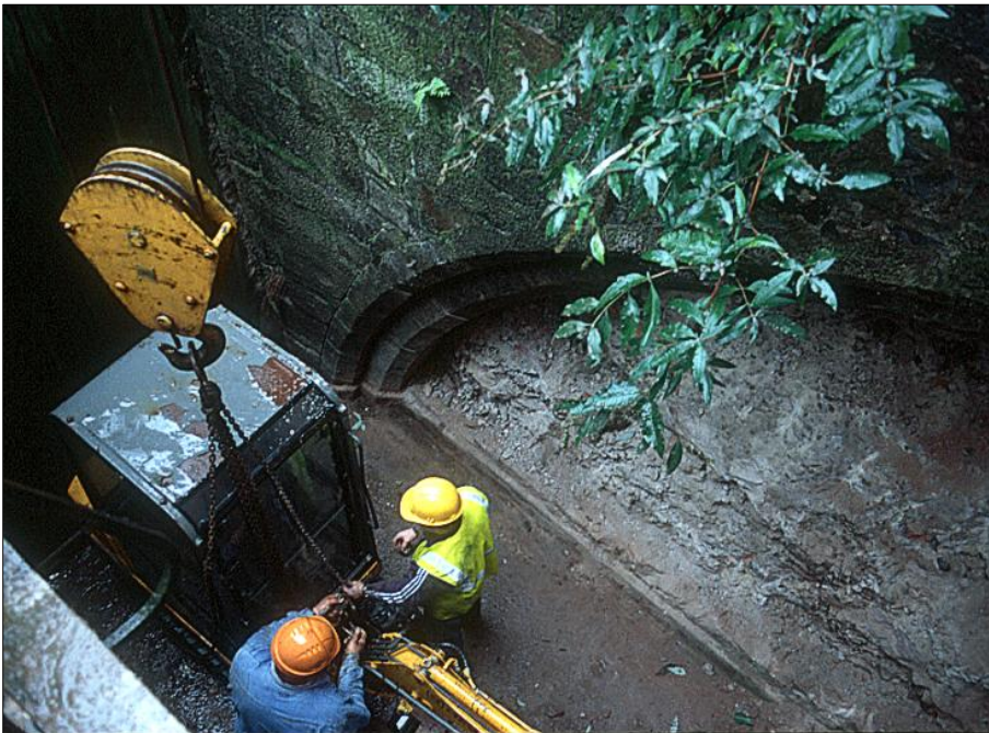
Ill B15: The eastern elevation of the bridge, looking into the inspection well for the north arch, and showing the concrete and brick infill of the arch revealed after removal of the brick facing.
