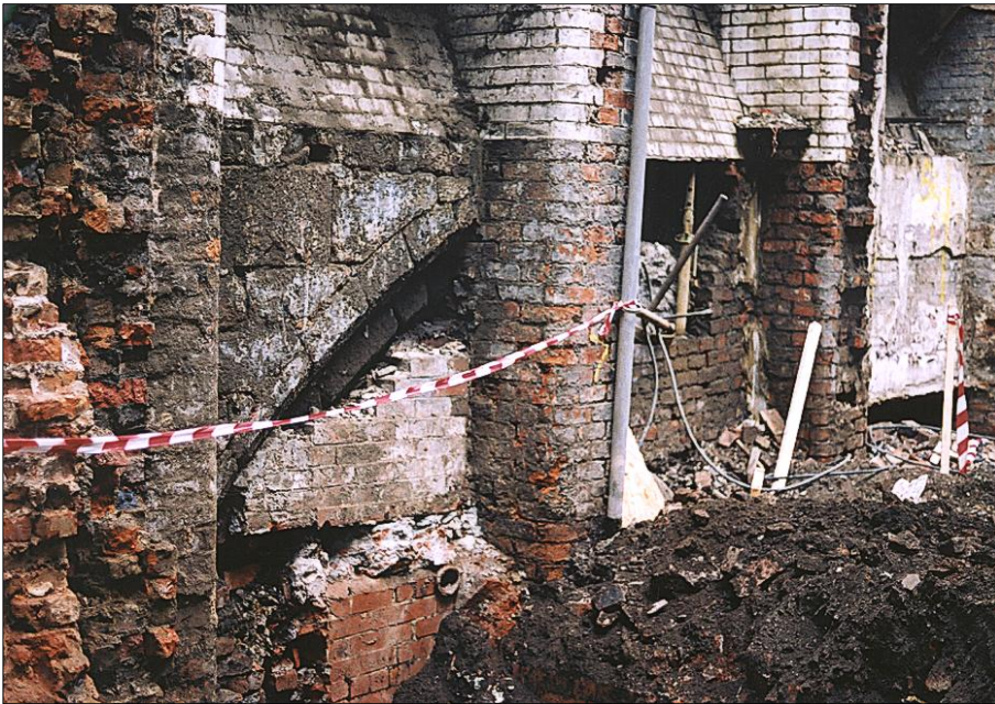
Ill B14: The eastern elevation of the bridge as exposed in the basement of Hanging Bridge Chambers, March 2001, showing the north arch.
