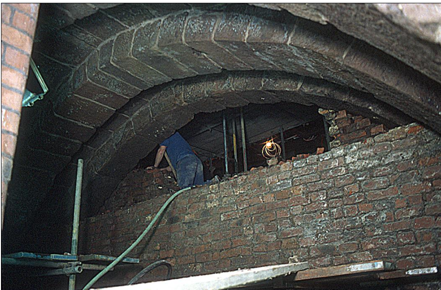
Ill B16: The southern arch, viewed through the basement of Mynshull's House during the removal of the brick wall blocking the eastern opening. Beyond the arch is the basement wall of Nos 10-12 Cateaton Street.
