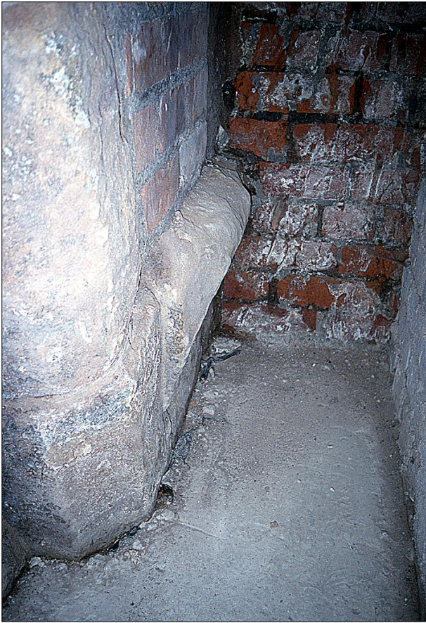
III B33: The west face of the central pier, showing the possible springer.
