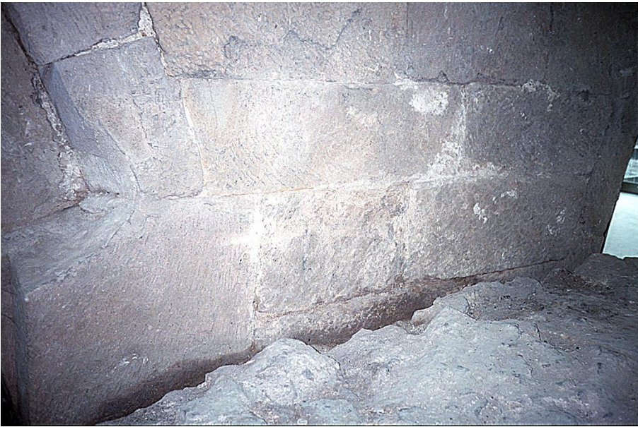
III B31: The east face of the central pier, showing surviving mortar between the courses.
