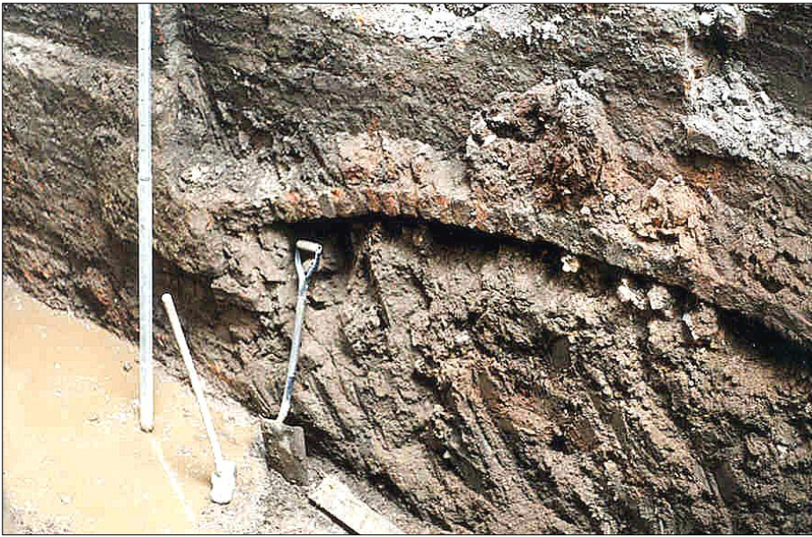
III B43: The lower part of the southern arch from the east, showing the brick retaining arch, presumably added in 1882 to support the west wall of Nos 10-12 Cateaton Street.
