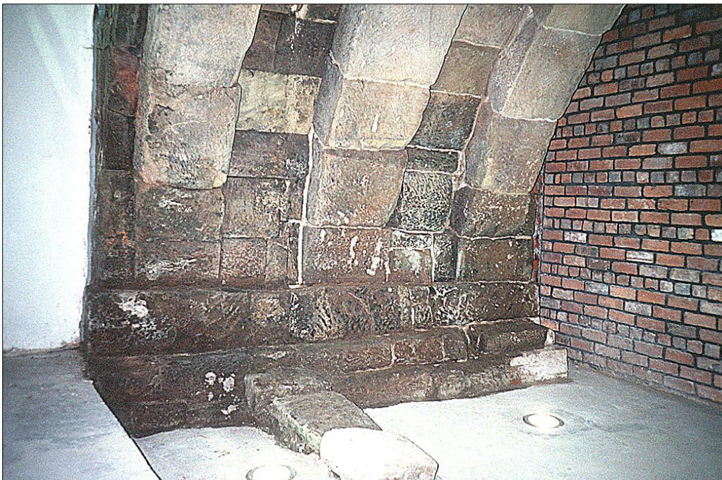
III B21: The south arch, the stepped base of the south side.
