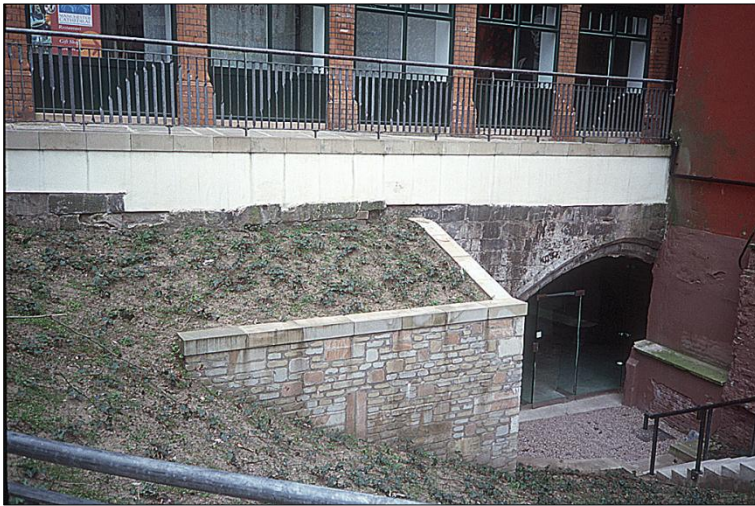
Ill B18: The western elevation of the north arch of the bridge viewed from Victoria Street.
